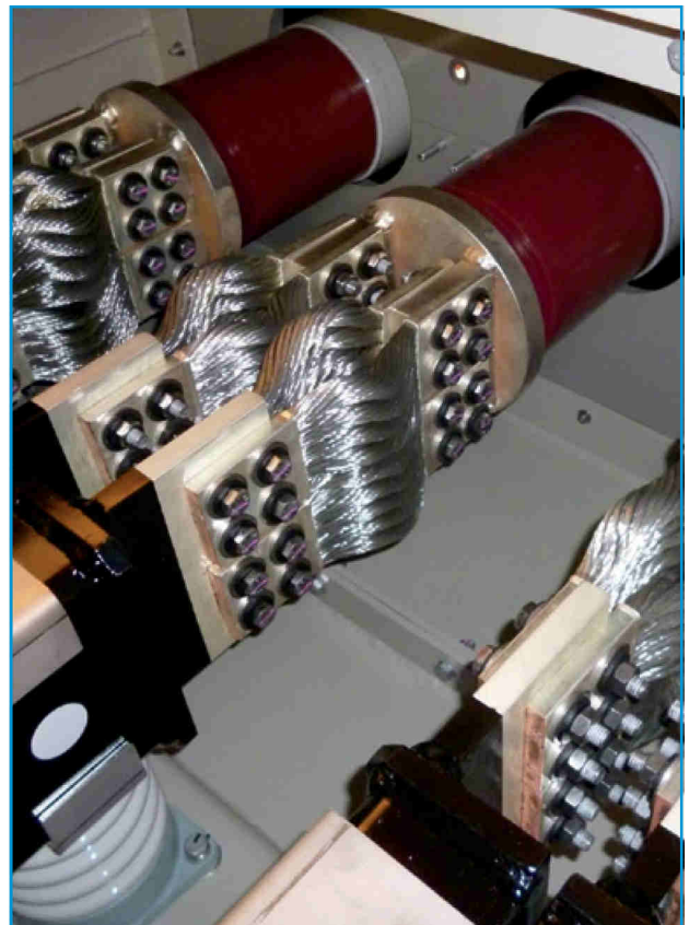
5000A generator connection
